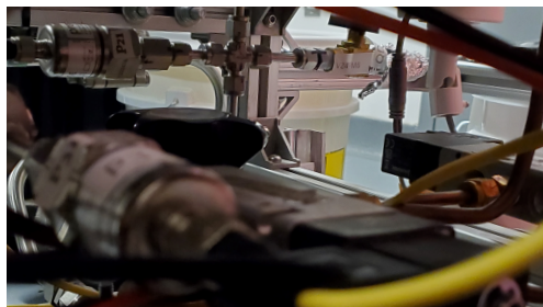
Figure 4.5.1.1: Pressure transmitters P31 and P21 installed
